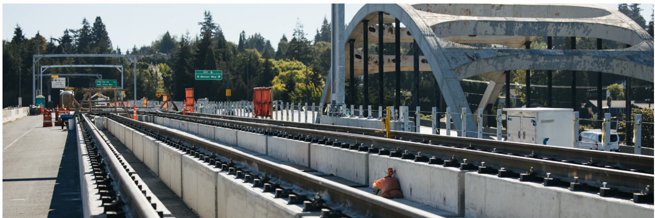
Construction of Sound Transit's Link light rail. Photo courtesy of Washington State DOT.
